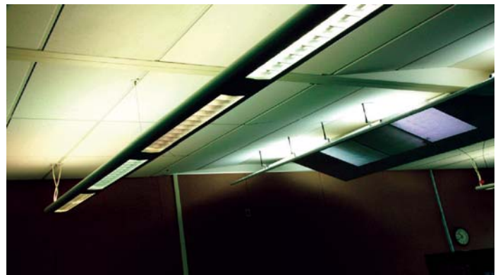
Direct-indirect lighting (left) and skylight reflectors (right) provide glare-free illumination.
