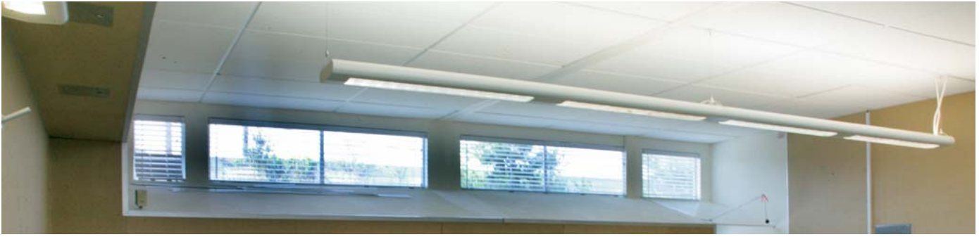
This interior elevation shows a light shelf and pendant mounted fixtures. The combination provides abundant light yet reduces glare.
