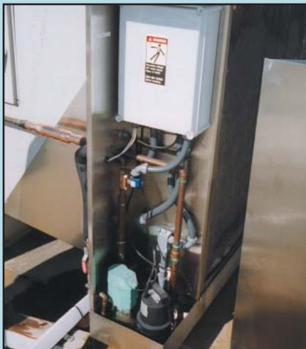
Cool water is passed through a heat exchanger to cool supply air without increasing its humidity.
