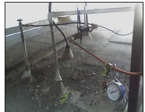
Figure 18: The water consumption for each of the units at ABC School was measured using Omega Engineering (FTB4605) in-line water flow meters with pulse output resolution of less than one ounce of water, a range of 0.15 to 20 gpm and an accuracy of +/-1.5%. Photo: ADM
