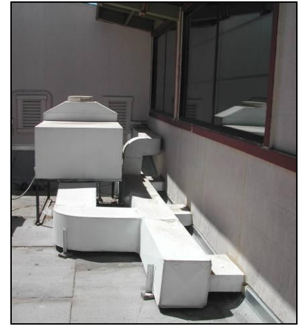
Figure 9: The original ductwork for the IDECs was very restrictive.
