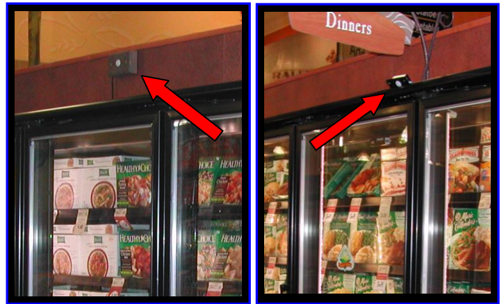
Figure 8: The prototype sensor (left) was mounted to a decorative façade above the freezer case. The final version of the sensor (right) was mounted directly to the frame of the freezer case.
