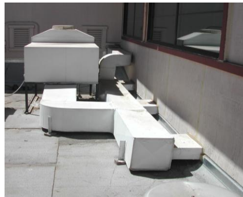
Figure 7: A poorly installed indirect-direct evaporative cooling system. The ductwork is far too restrictive to deliver the airflow needed to meet the cooling requirements of this classroom. 6
