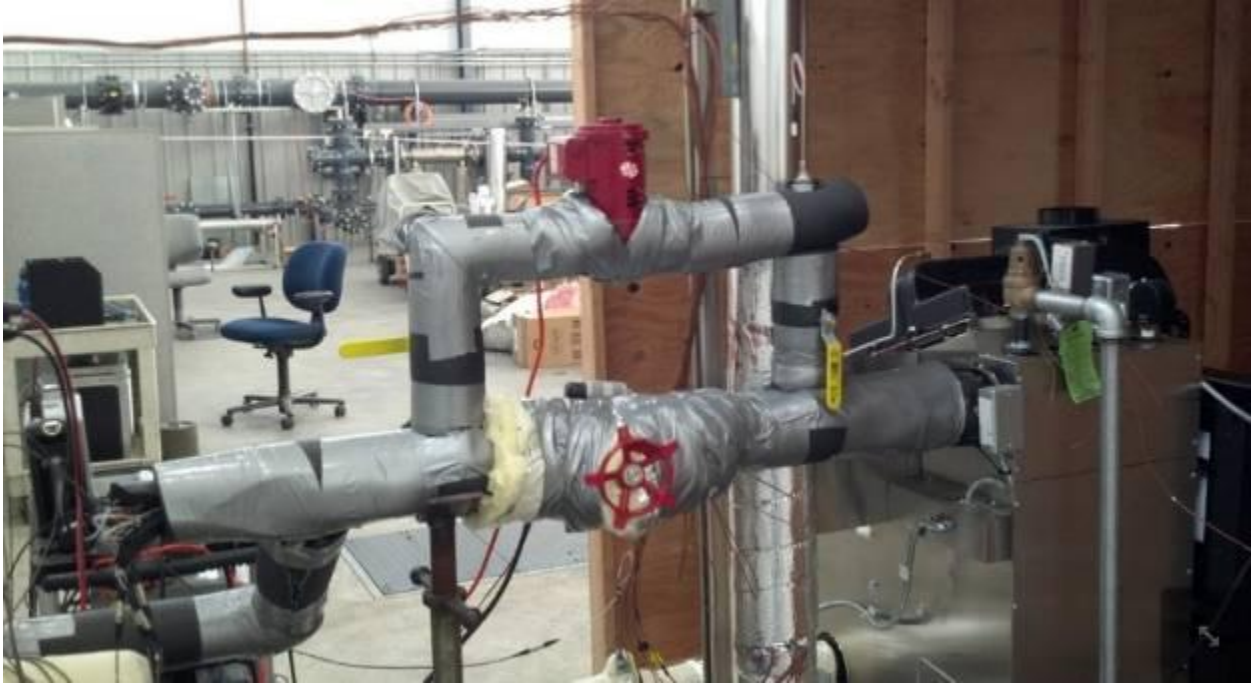
FIGURE 36: STRATIFICATION MITIGATION – INSTALLED SOLUTION
