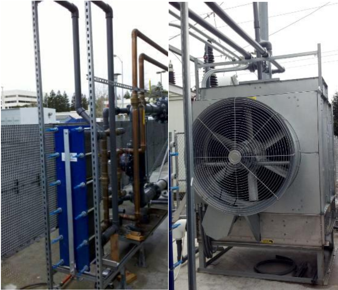
FIGURE 5. TEST APPARATUS – HEAT EXCHANGER AND COOLING TOWER
