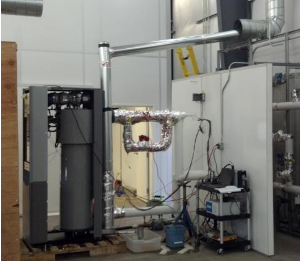
FIGURE 7. UNIT 3 FLUE DUCT TO PREVENT OVERSPRAY OF FLUE CONDENSATE
