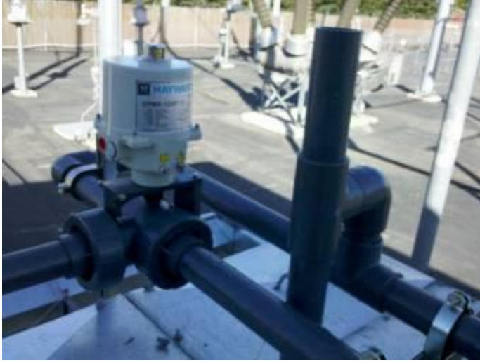
FIGURE 6. TOWER 3-WAY MIXING VALVE AND BYPASS SYSTEM
