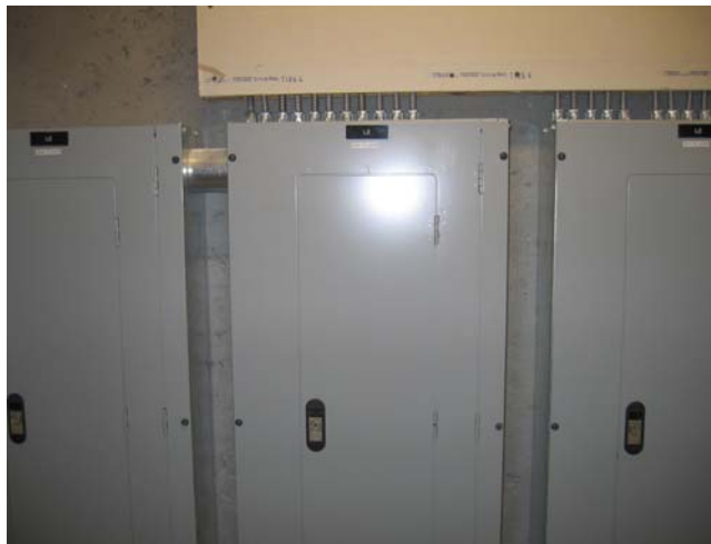
Figure 7: Electrical Panels in Hotel #1
