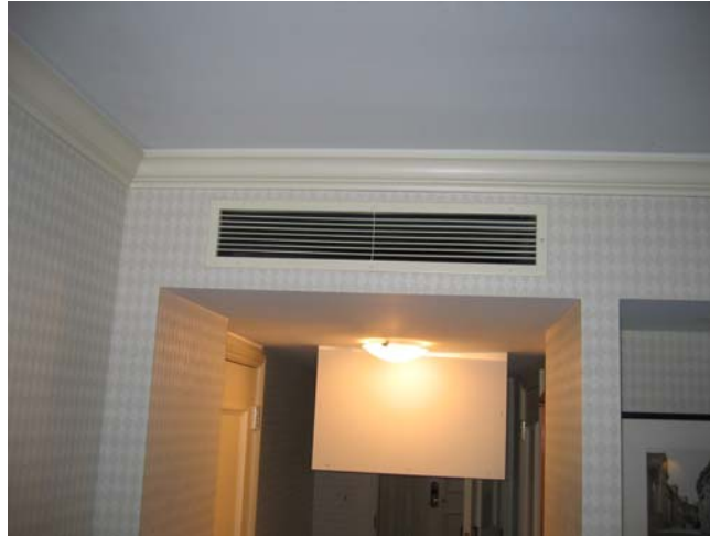
Figure 16: Hotel #2 Supply Air Grill
