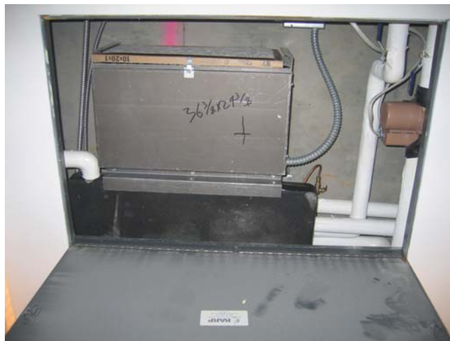
Figure 15: Hotel #2 Fan Coil Unit
