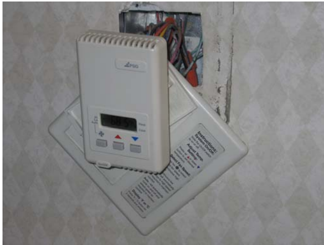
Figure 11: Room Thermostat in Hotel #2
