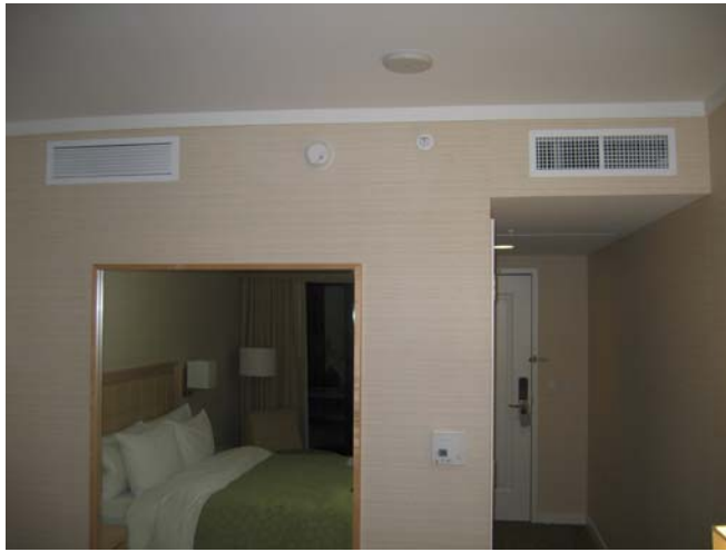
Figure 6: Hotel #1 Guestroom Supply Air and Return Air Grills
