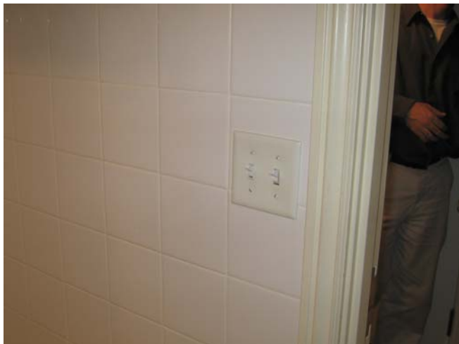
Figure 12: Bathroom Light Switches in Hotel #2
