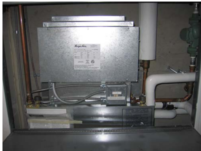
Figure 5: Hotel #1 Fan-Coil Unit
