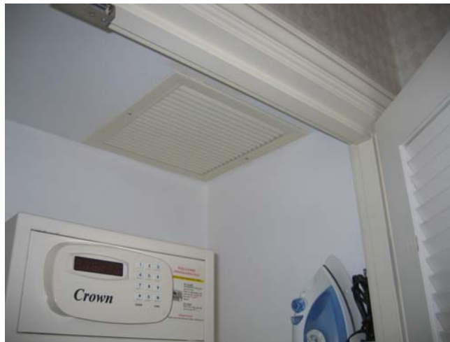
Figure 17: Hotel #2 Return Air Grill
