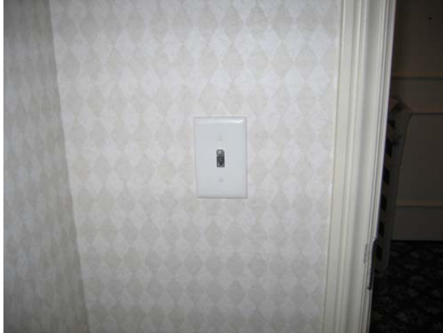
Figure 10: Main Light Switch in Hotel #2
