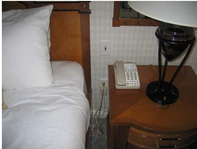
Figure 13: Electrical Outlets in Hotel #2
