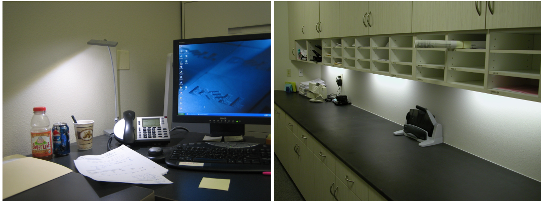
Figure 11. Task Lighting After Retrofit
