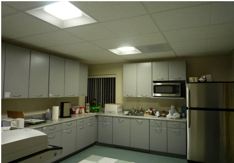
Figure 7: LED Troffer in Kitchen Area
