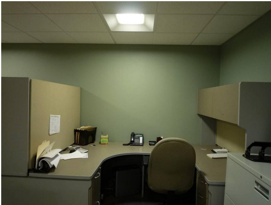
Figure 1: LED Troffer in Open Work Space
