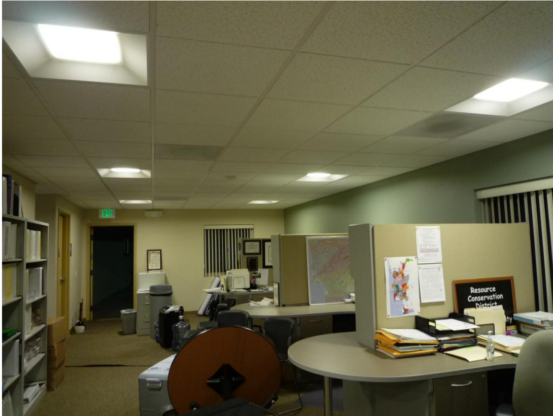
Figure 6: LED Troffers in Open Office Area
