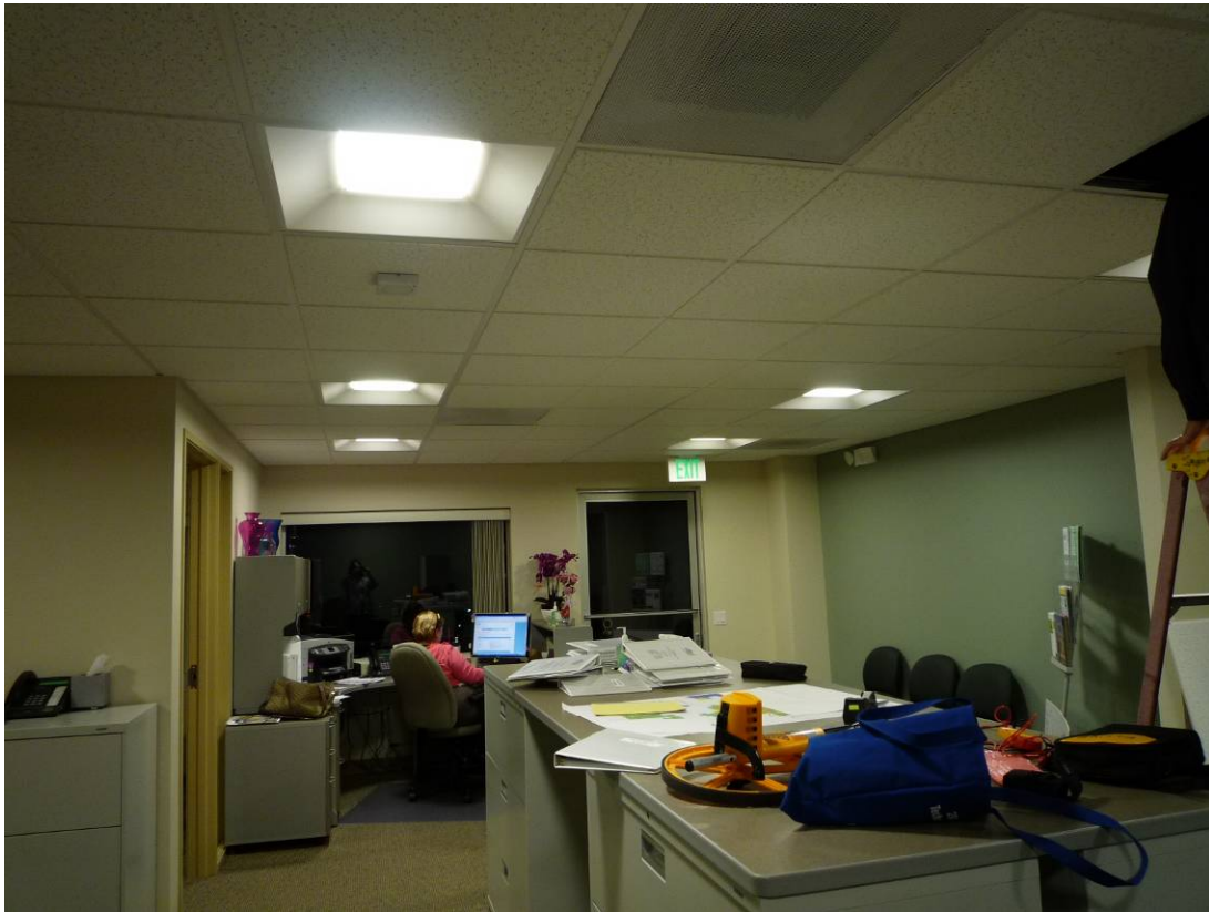
Figure 6: CREE LR24 LED Troffers In Open Office Area
