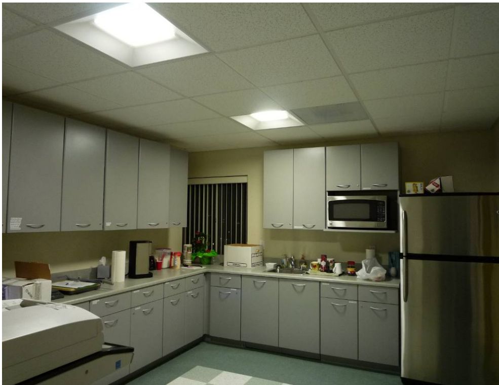
Figure 7: CREE LR24 LED Troffer in Kitchen Area
