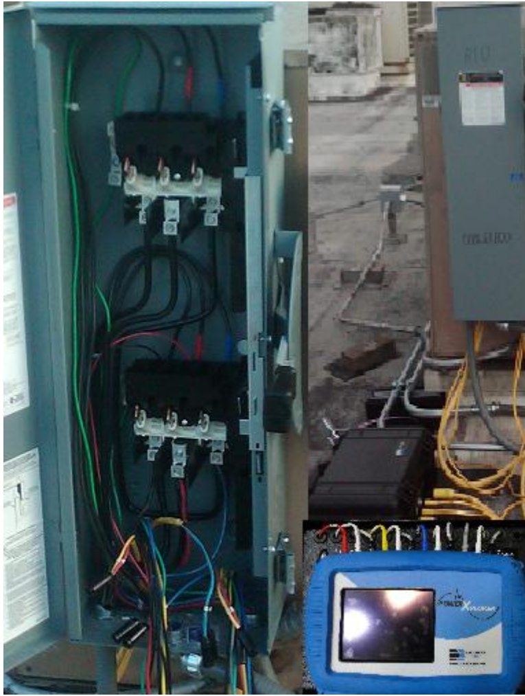
FIGURE 2 ELECTRICAL SETUP AT TEST SITE
