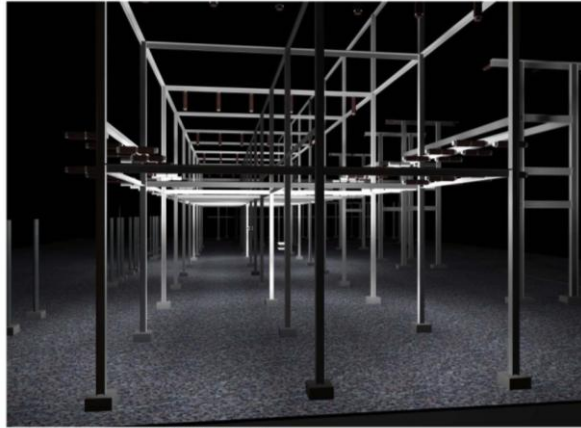
250W PULSE START METAL HALIDE at REDLANDS SUBSTATION
