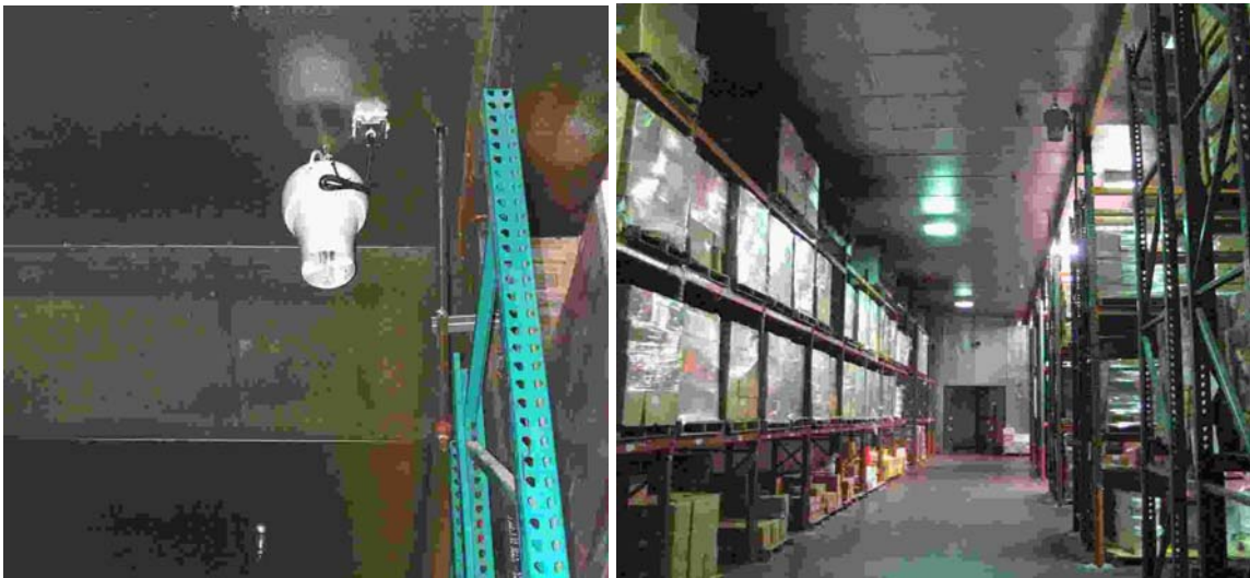
FIGURE 12. DESTRATIFICATION FANS INSTALLED IN COOLER
