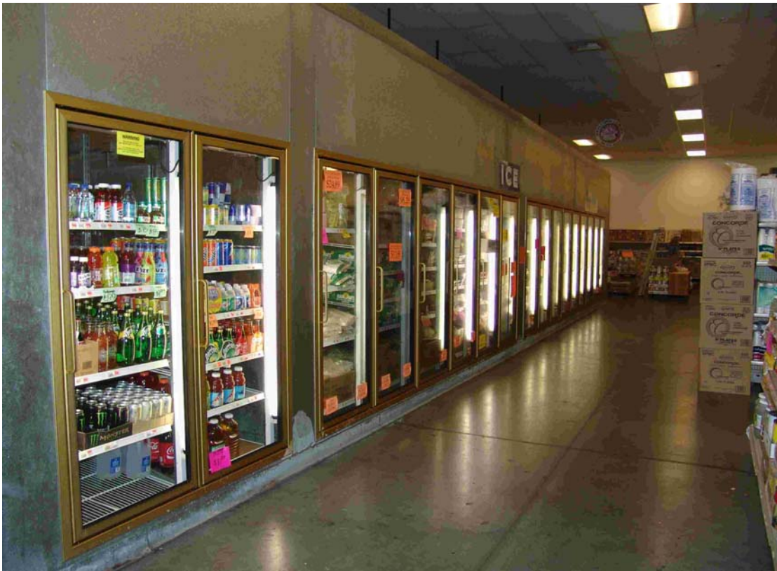
FIGURE 10. RETAIL COOLERS AND FREEZER
