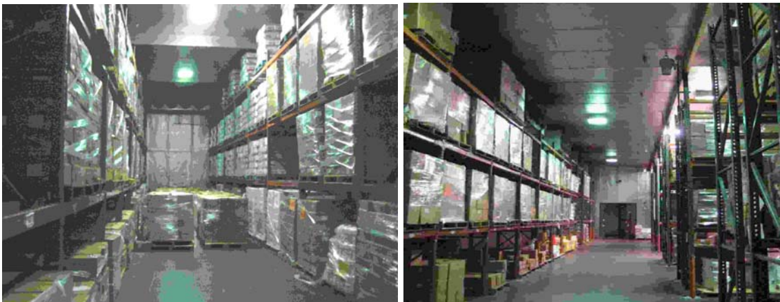
FIGURE 8. INSIDE MEDIUM TEMPERATURE COOLER
