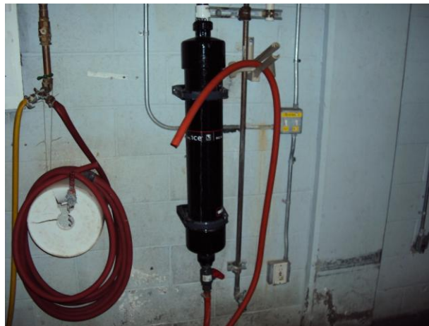
FIGURE 4. INSTALLED REALICE SYSTEM
