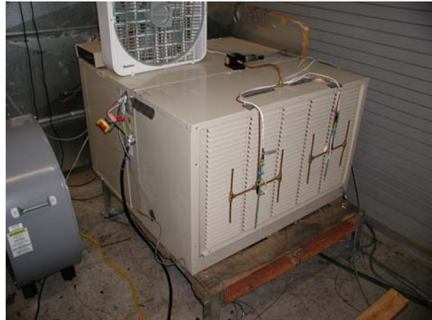
Figure 5: ECU2 under Test
