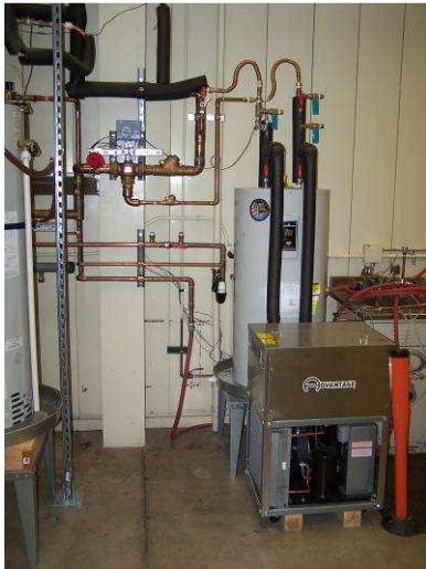
Figure 3: Water Tempering System
