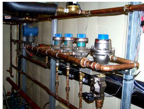
Figure 4: Flow Control Valve Array and Mass Flow Meter
