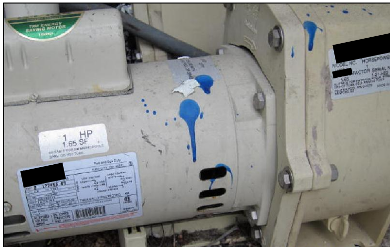
Figure 4: (BASELINE) Single Speed Pool Filtration Pump
