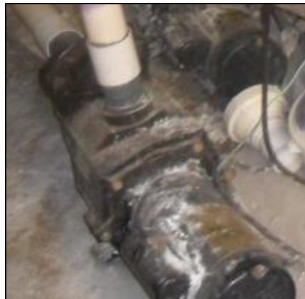
Figure 10: (BASELINE) Single Speed Spa Filtration Pump (Pool Pump Similar)
