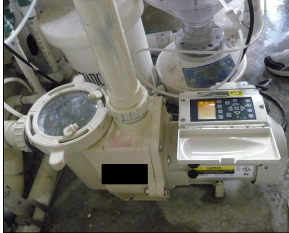
Figure 11: (RETROFIT) Variable Speed Pool Filtration Pump Tested (Spa Pump Similar)
