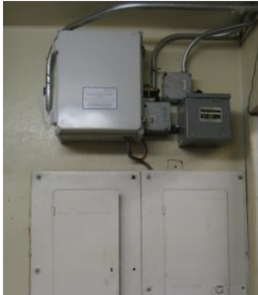
FIGURE 2. K20 POWER LOGGER MOUNTED NEXT TO ELECTRIC PANELS
