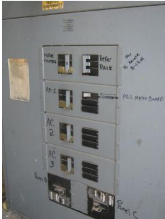
FIGURE 3. AIR CONDITIONER BREAKERS IN ELECTRIC ROOM
