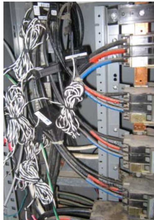
FIGURE 4. CURRENT TRANSDUCERS MOUNTED INSIDE ELECTRIC PANEL
