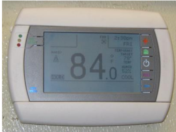
FIGURE 1. PCT MOUNTED ON WALL
