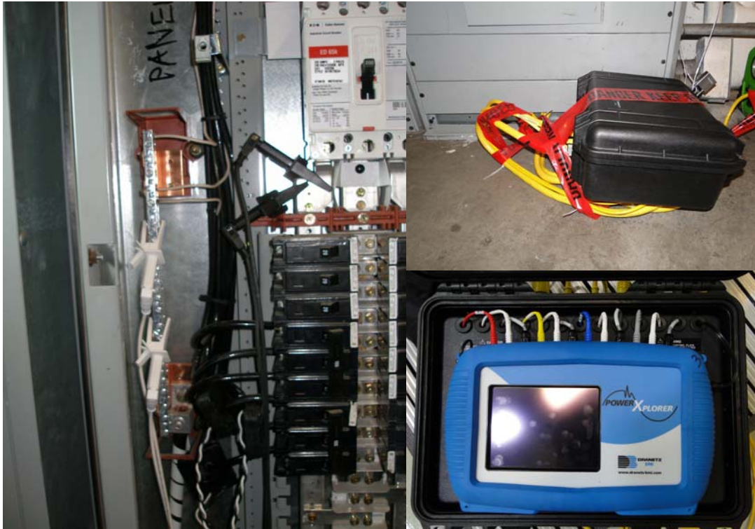
FIGURE 7. FIELD MONITORING EQUIPMENT SETUP
