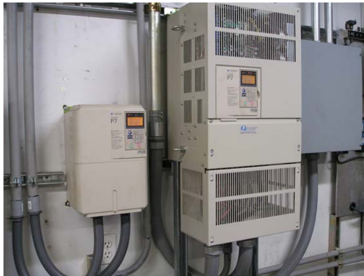
FIGURE 5. VARIABLE SPEED DRIVE WITH A KEYPAD MOUNTED ON FRONT
