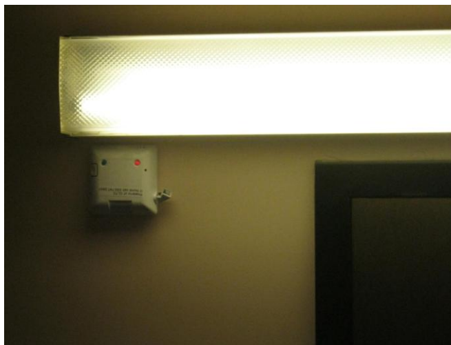
FIGURE 5: OCCUPANCY LOGGER IN STAIRWELL
