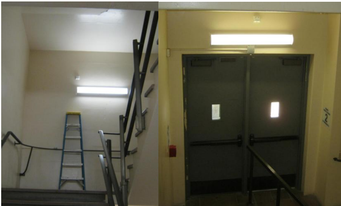
FIGURE 23. OCCUPANCY LOGGERS IN STAIRWELL
