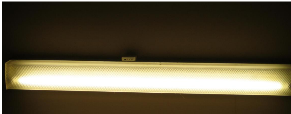
FIGURE 4: STAIRWELL LIGHT FIXTURE WITH LIGHTING LOGGER
