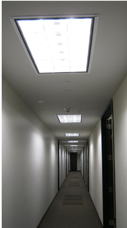
FIGURE 2: 10TH FLOOR BASELINE CORRIDOR LIGHTING
