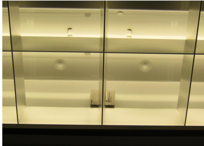
FIGURE 3: CORRIDOR CEILING LIGHT FIXTURE WITH LIGHTING LOGGER
