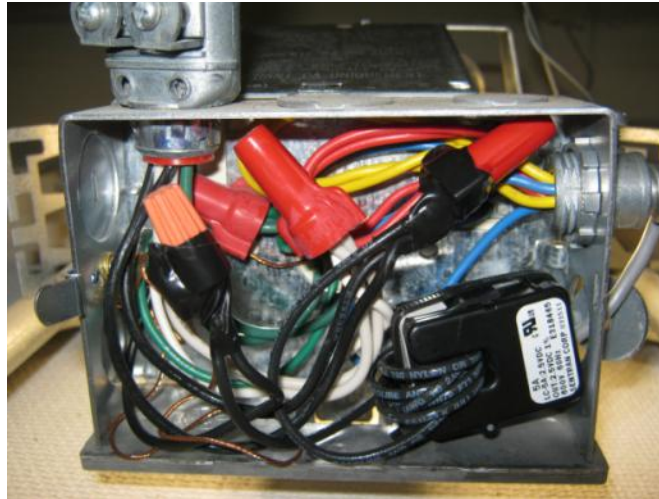
FIGURE 19. CURRENT TRANSFORMER USED TO MONITOR THE BASELINE CORRIDOR LIGHTING
