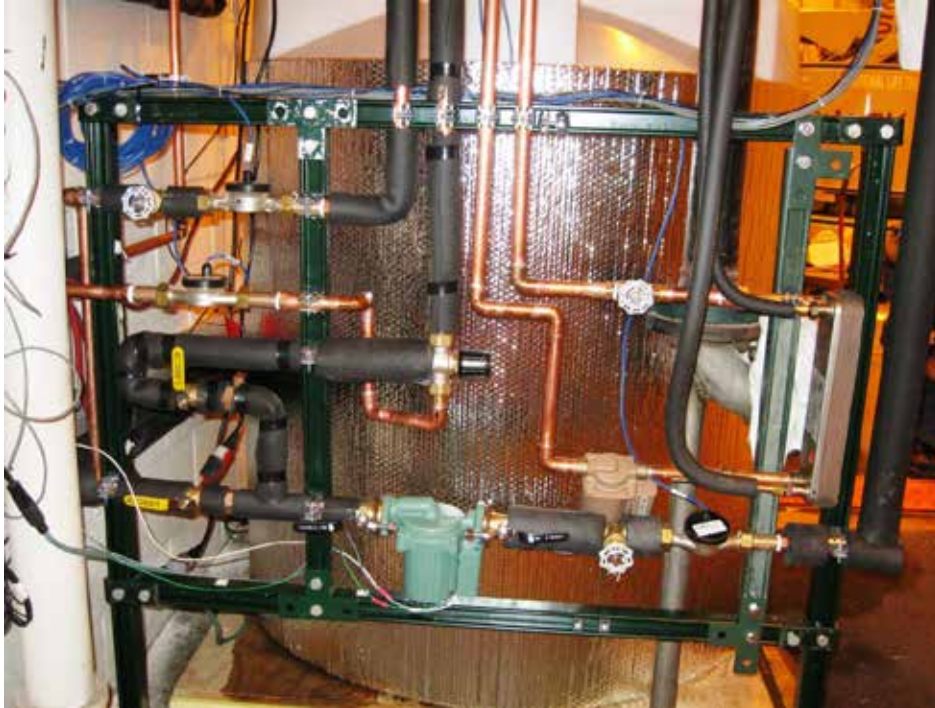
Figure 2 Chilled Water Storage Tank (Background): Plumbing System and Chilled Water Heat Exchanger (Foreground)
