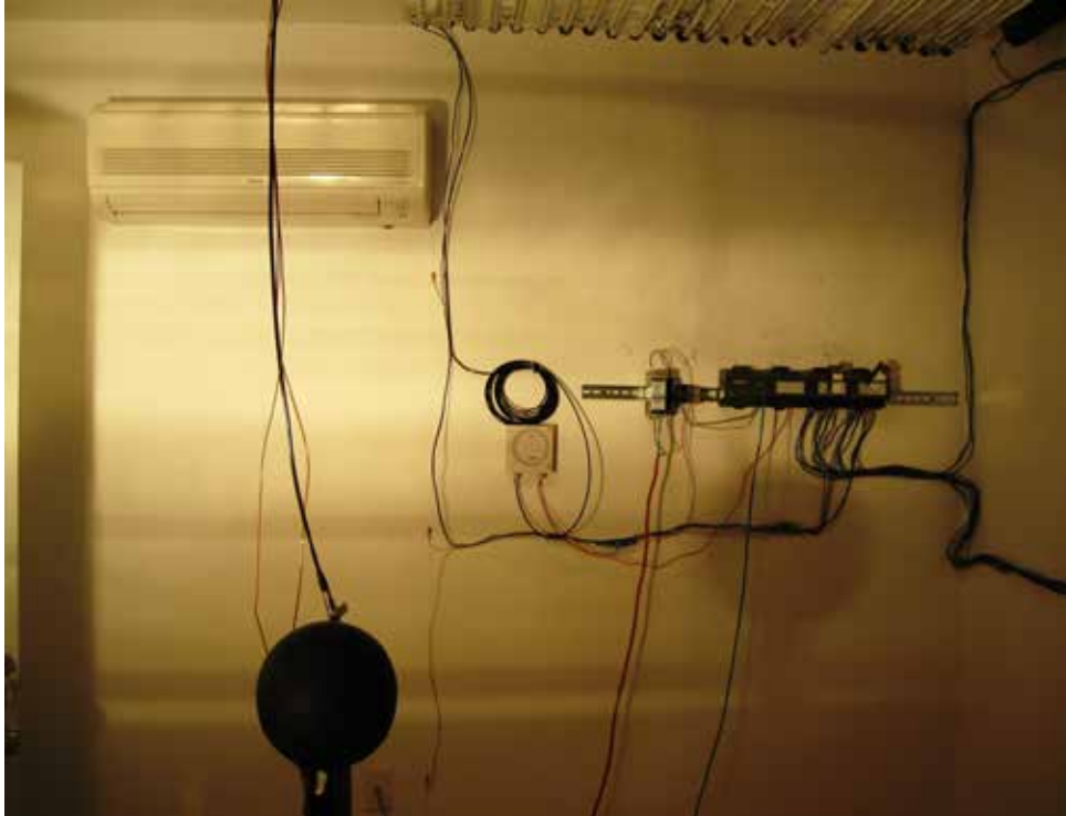
Figure 5 MRT Globe, RH Sensor, Wall-Mounted Thermocouples, and Labview Fieldpoint Modules
