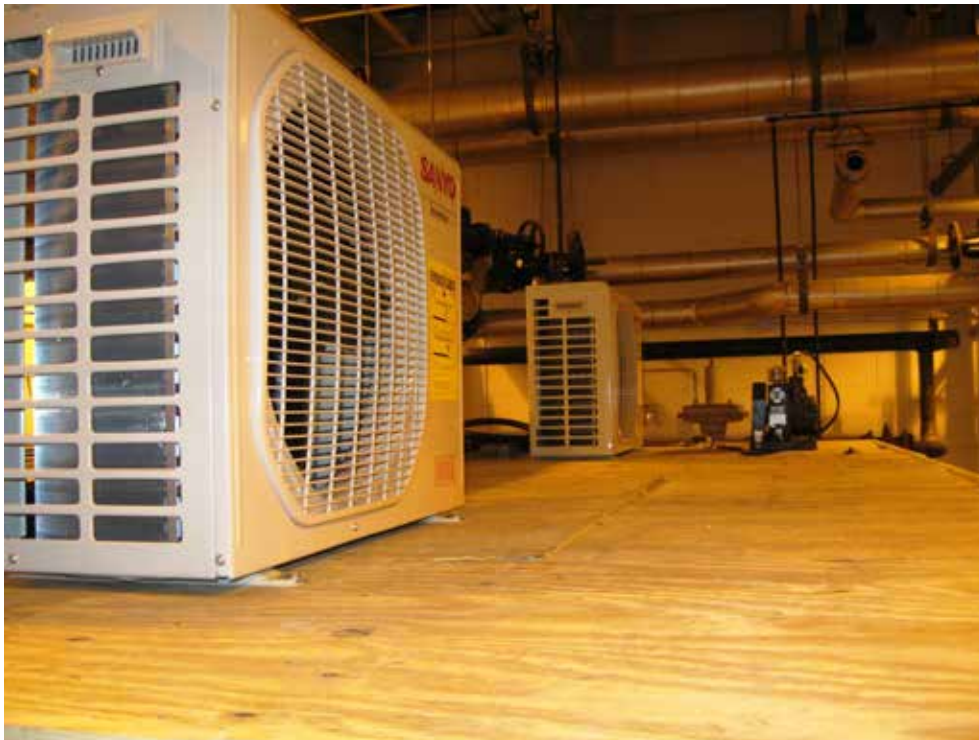
Figure 3 Mini-split Heat Pump (Foreground); Mini-Split Chiller for Chilled Water Production (Background)
