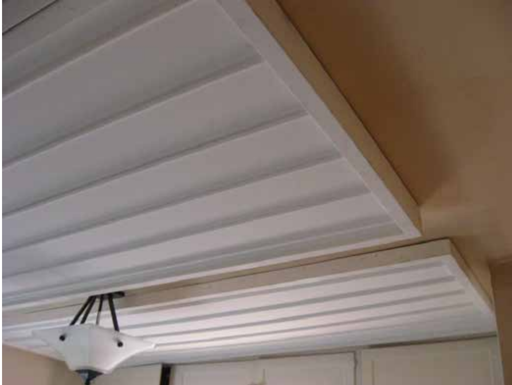
Figure 19 Radiant panels installed in the 6th Avenue house
