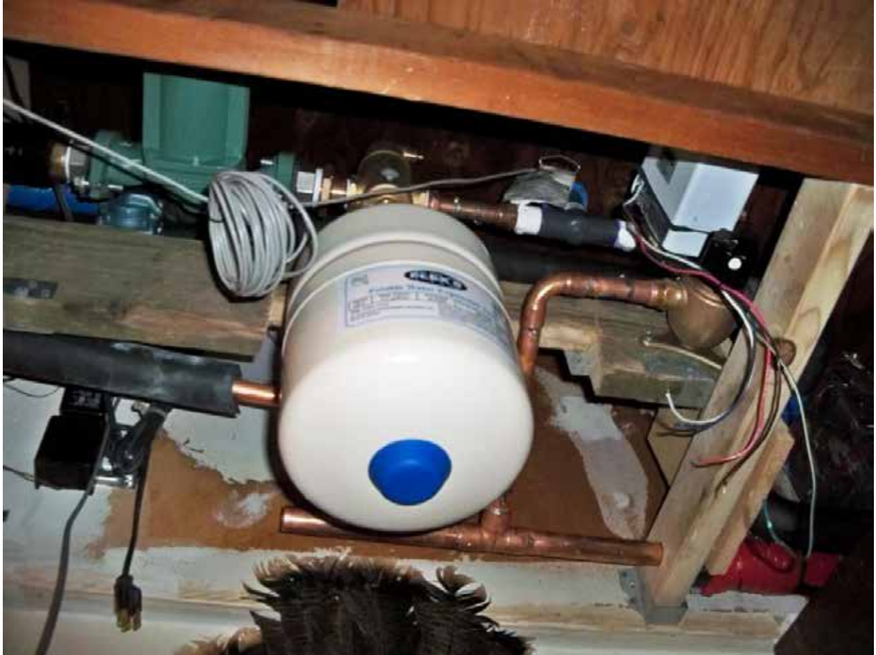
Figure 14 Hydronic system in Grandstaff house
