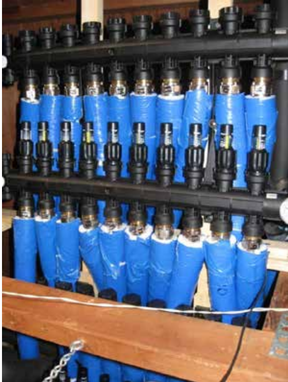
Figure 13 Uponor piping manifold in Grandstaff house
