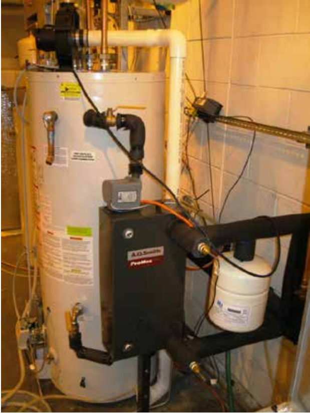
Figure 17 High efficiency water heater in the lab showing with side mount heat exchanger
