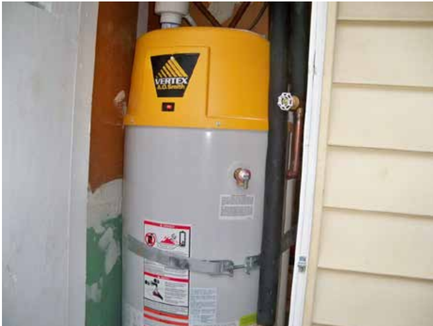
Figure 16 High efficiency water heater installed in Grandstaff house
