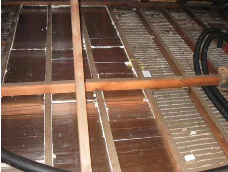
Figure 21 Measured Home Performance installation in 6th Avenue house
