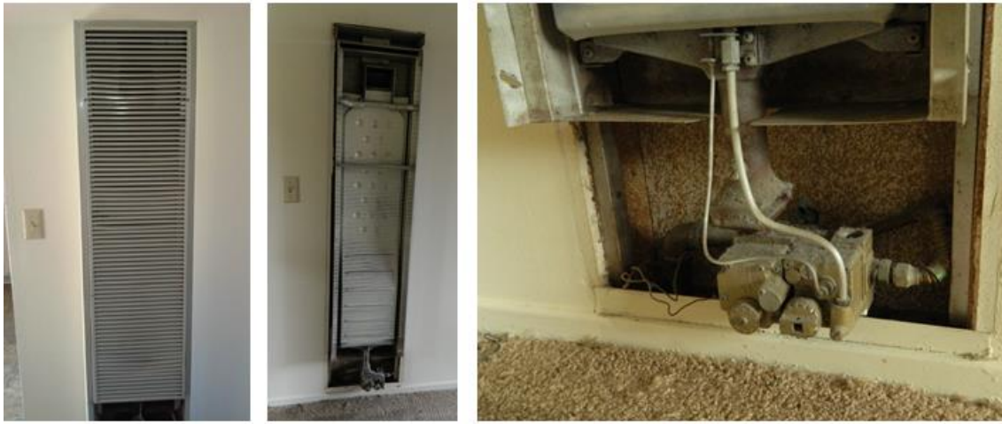
Original wall furnace with heat exchanger and pilot light igniter
