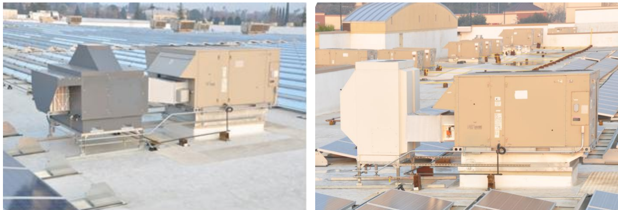
FIGURE 3. PHOTOS OF COMPLETE INSTALLATION FOR TYPE C (LEFT) AND TYPE M (RIGHT) INDIRECT EVAPORATIVE AIR CONDITIONERS. SIX ROOFTOP UNITS WERE RETROFIT, THREE WITH EACH EQUIPMENT TYPE
