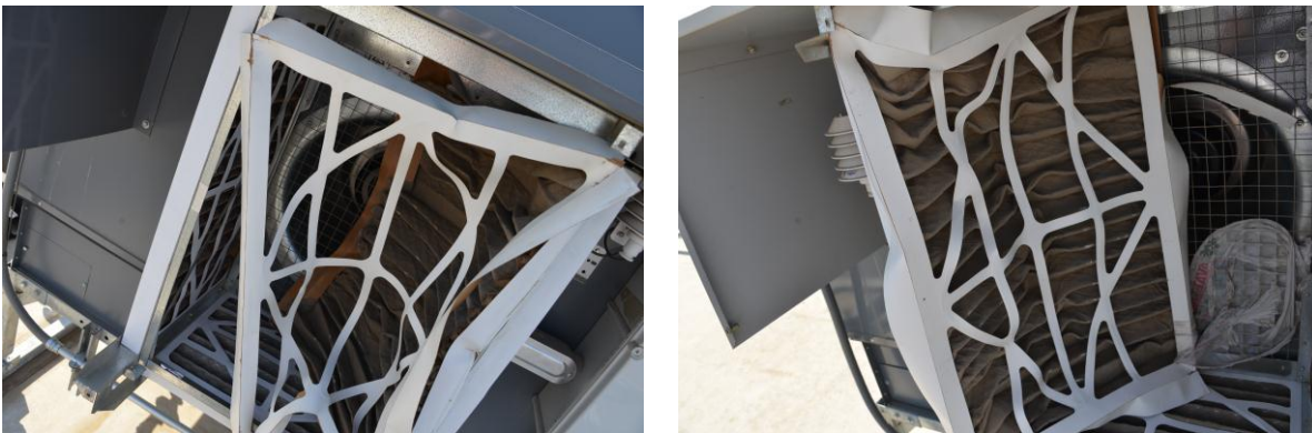
FIGURE 6. FILTERS REQUIRE REPLACEMENT EVERY 30 DAYS OR ELSE AIR-FLOW WILL BE RESTRICTED AND MAY LEAD TO FILTER FAILURE AND DEGRADED SYSTEM PERFORMANCE
