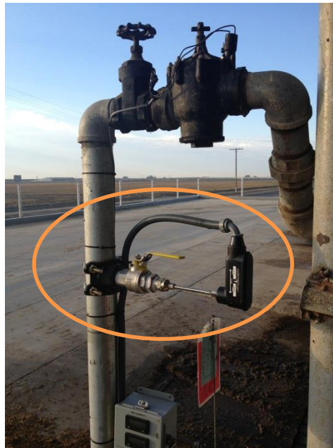
FIGURE 4. A FLOW METER INSTALLED ON THE SOAKER LINE WATER SUPPLY LINE
