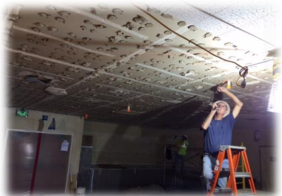
Figure 2: Removal of ceiling tiles was a daunting task when it was found they were glued to the ceiling and the old glue had to be chiseled off.
