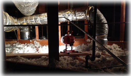
Figure 3: The new lighting system required installing new structural supports, electrical conduit, electrical outlet boxes and control wires. All of this work had to be performed above the ceiling in an insulated attic.
