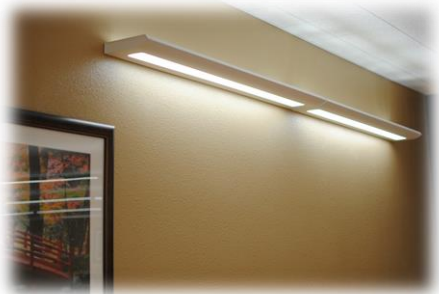
Figure 7 Philips BoldPlay indirect/direct LED fixtures (wall mounted)
