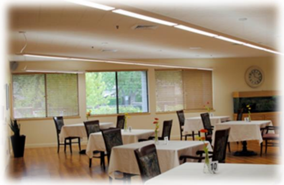
Figure 1: The new lighting system included state-of-the-art suspended LED fixtures with indirect-direct lighting distribution and touchpad controls
