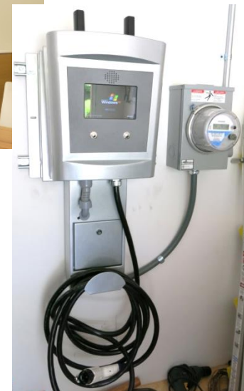
Electric Vehicle Charging Station
