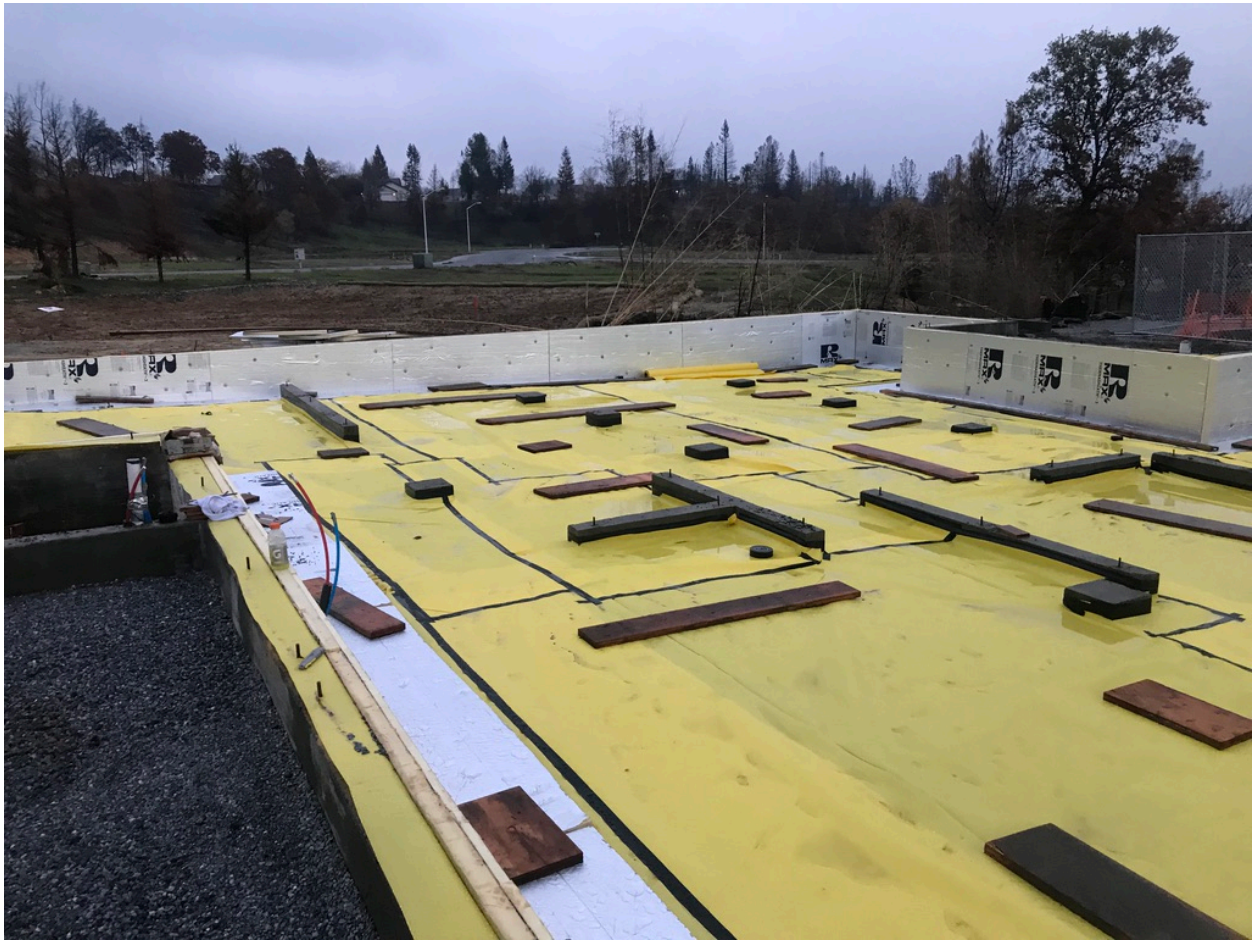
FIGURE 2: CRAWLSPACE PERIMETER INSULATION AND SEALED VAPOR BARRIER
