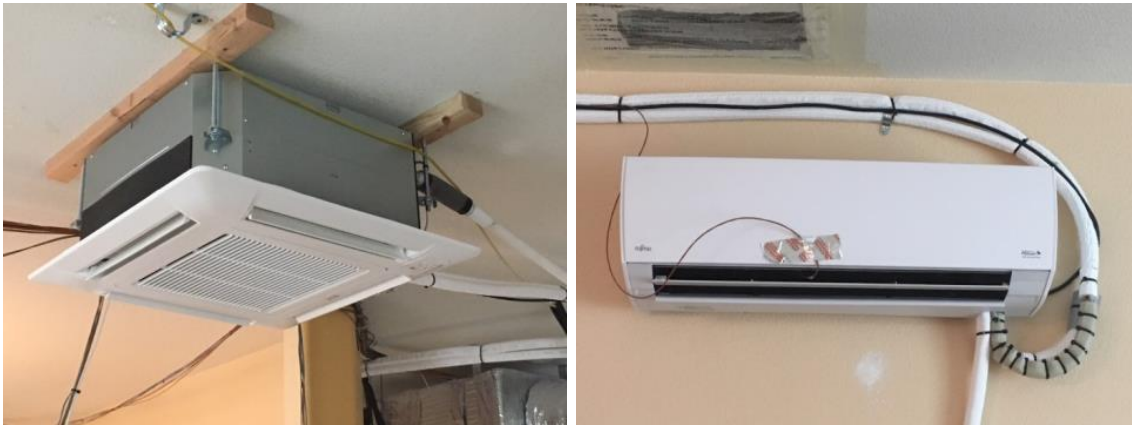
FIGURE 10. DUCTLESS VCHP INDOOR UNITS: CEILING UNIT IN DINING ROOM (LEFT), AND WALL UNIT IN LIVING ROOM (RIGHT)
