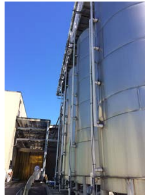
Fermentation Tank Chilled Water Piping
