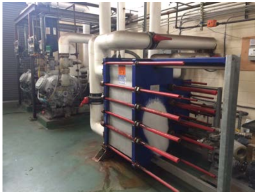
Existing R-22 Chiller System Engine Room location
