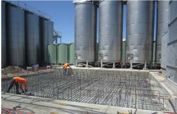
New Process Tank and Mechanical Pad
