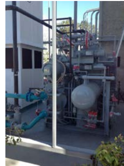
Factory Package and Tower
