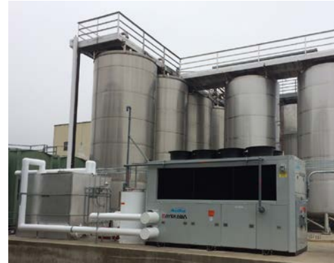
New NH 3 Chiller and CHW Tank
